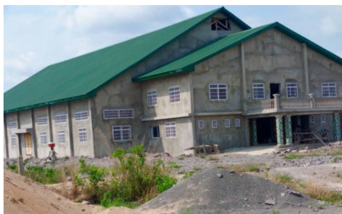
District office of the Sierra Leone People's Party (SLPP) being constructed by the Koidu Limited Mining Company. Kono district.
