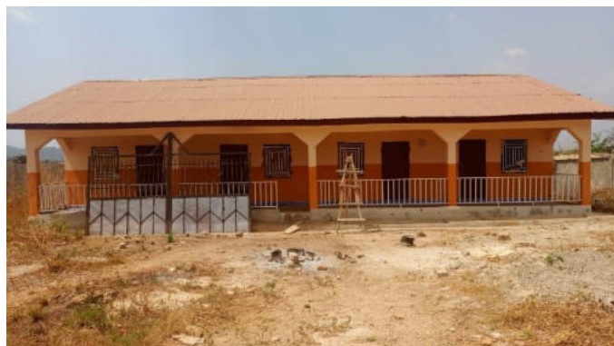
Abandoned Quarters for nurses constructed from the CDAP Fund at Komoro, Nimikoro Chiefdom.
