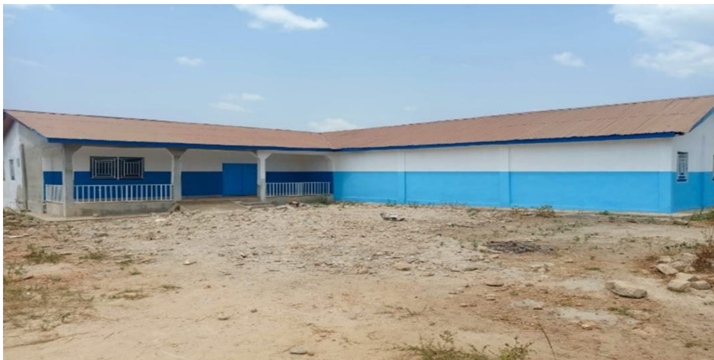
Abandoned Health Centre constructed from the CDAP Fund at Komoro, Nimikoro chiefdom.
